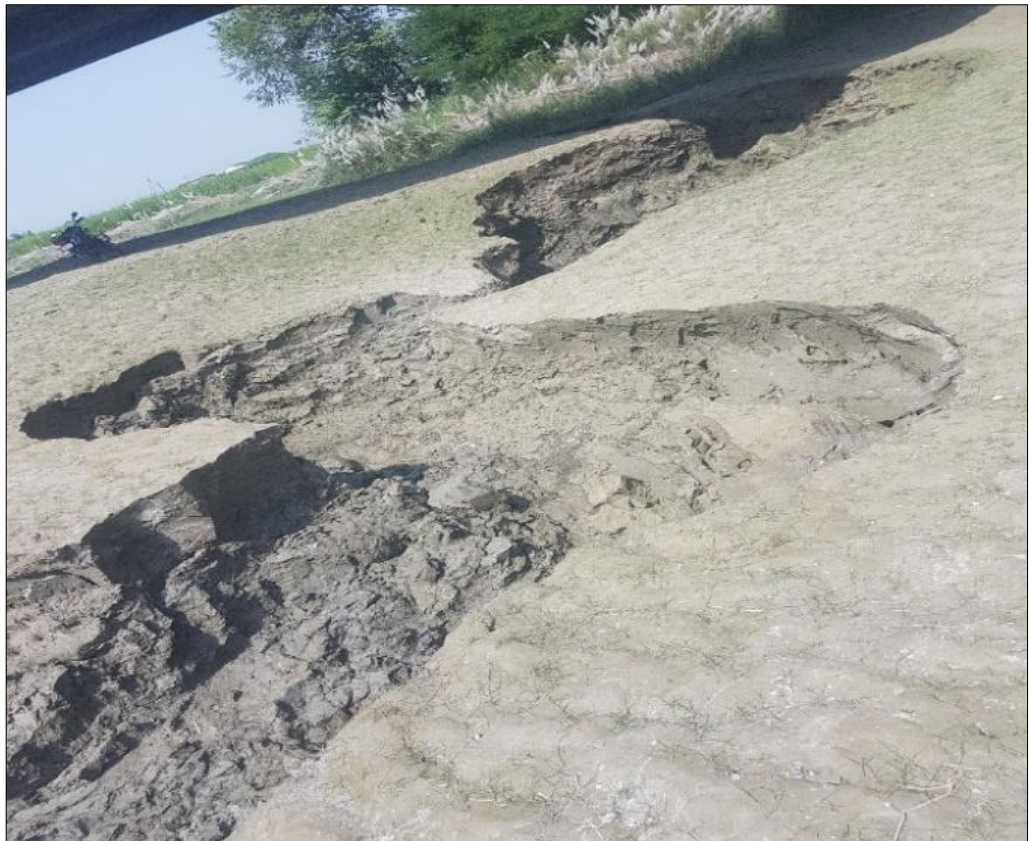
Figure 5-20 Kosi River scouring (Picture was taken during the field visit in October 2018)
