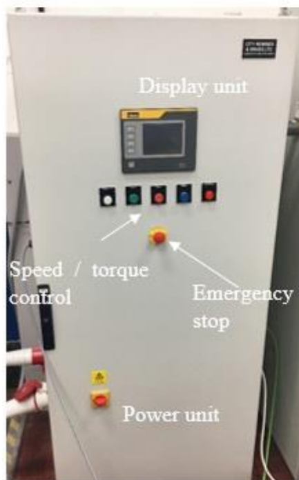
(e) Speed control panel
