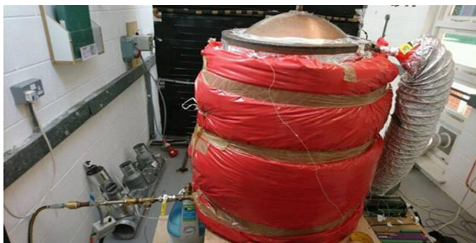
Figure 9.11. The humidifier and the air heater connections
