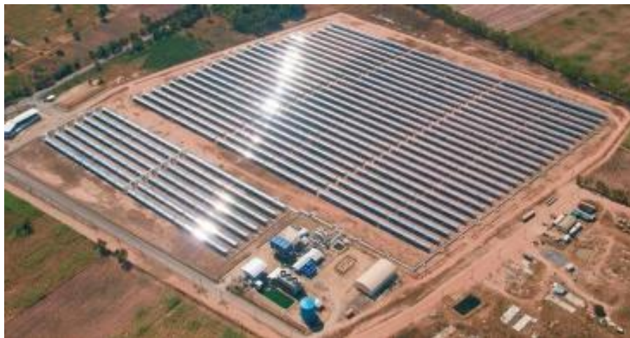
Figure 3.12: Aerial view of TSE1, Kanchanaburi, Thailand [98]
