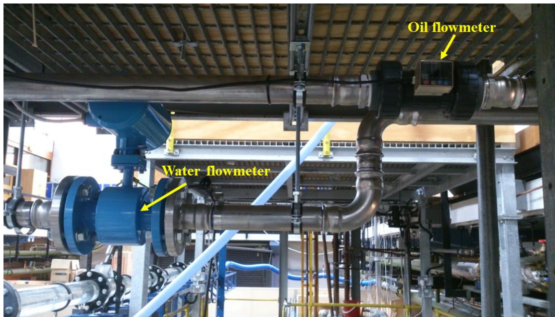
Figure 4-10 Photograph of both flow meters in place for flowrate measurements
