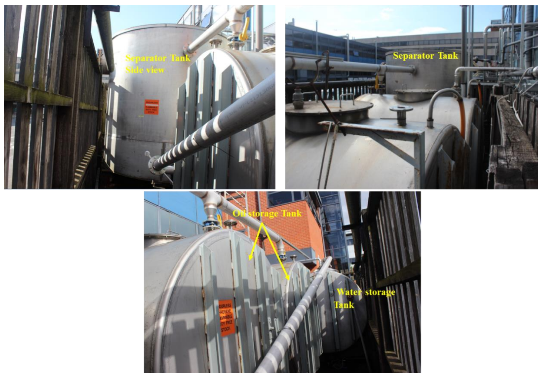
Figure 4-2 Liquid Storage Tanks and Separator vessel
