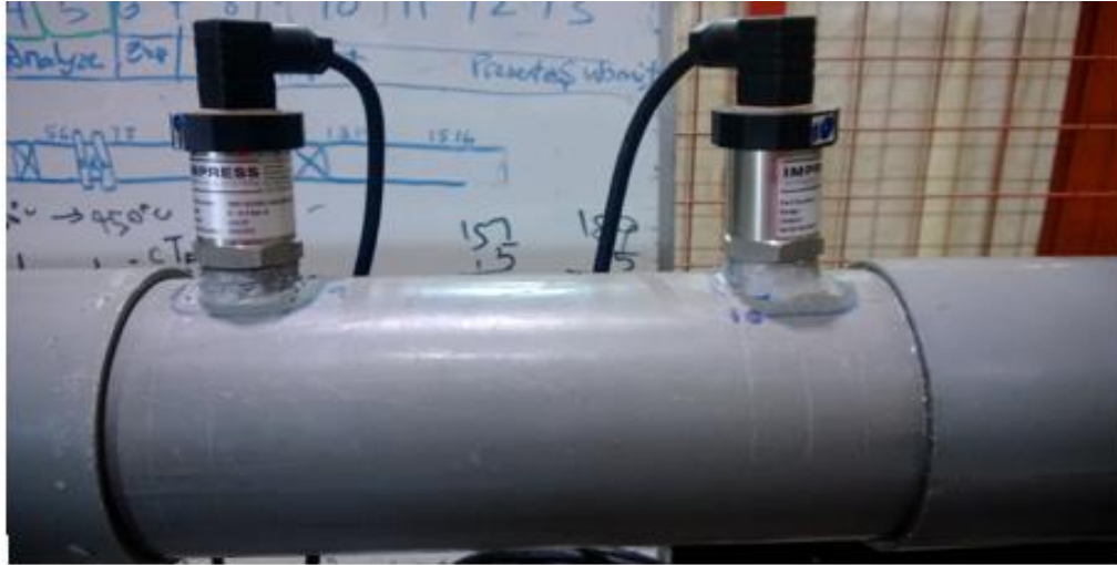
Figure 3.3: The Pressure Sensor pairings flush mounted to PVC pipe sections.
