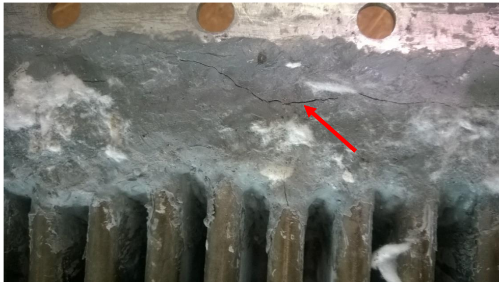
Figure A2: Crack on the gasket sealings.
