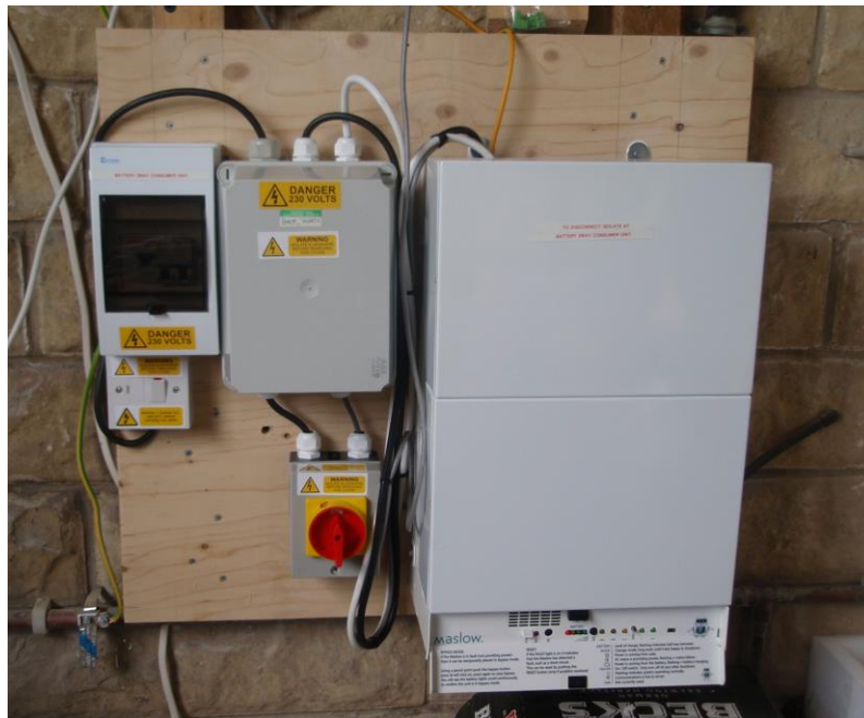
Figure 3.3: 2 kWh 0.5 kW Moixa Maslow batteries installed on one of the four properties of Corsham Trial.
