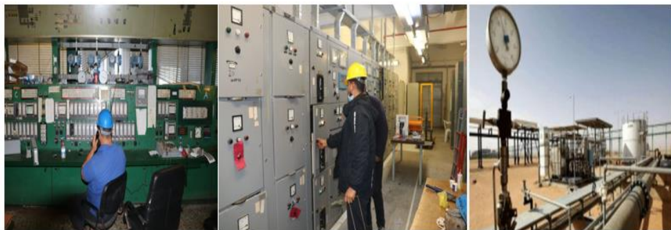
Figure 6. 3 Photos of the control room and data record room in the oil refinery.
